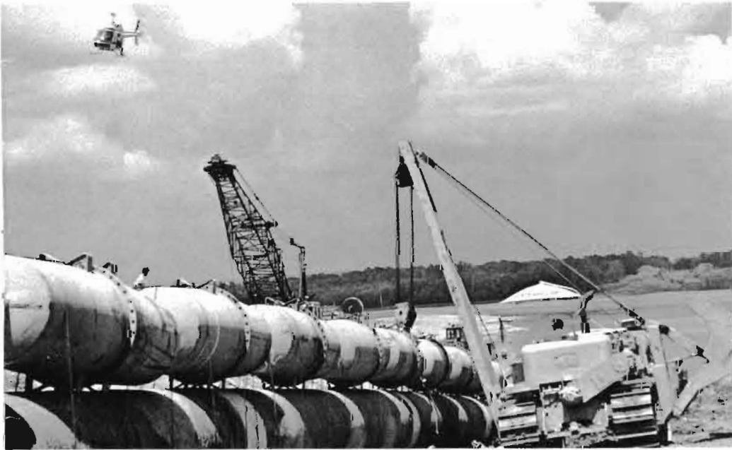
Capline spans the Ohio. pontoons buoy up the 26-ton, concrete-coated sections as they are pulled across the river by cable.
