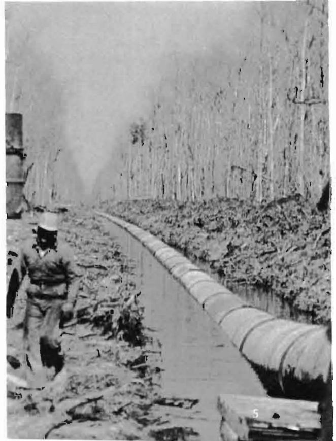
Pipe without the concrete wrap is buoyant enough to be joined and pushed ahead in this water-filled ditch.
