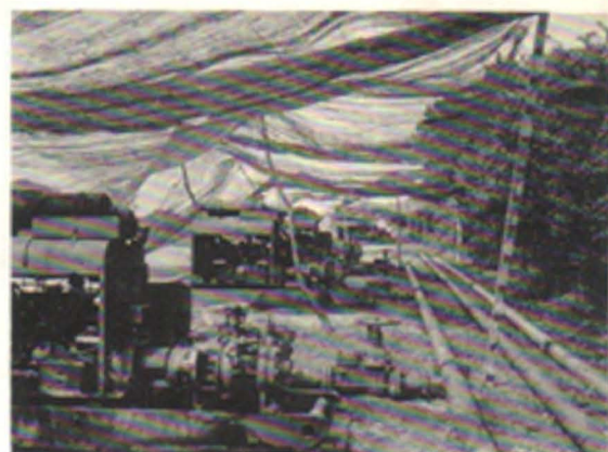
There were 72 portable pumping stations on the Northern Pipe Line System from Cherbourg to the Rhine River.
