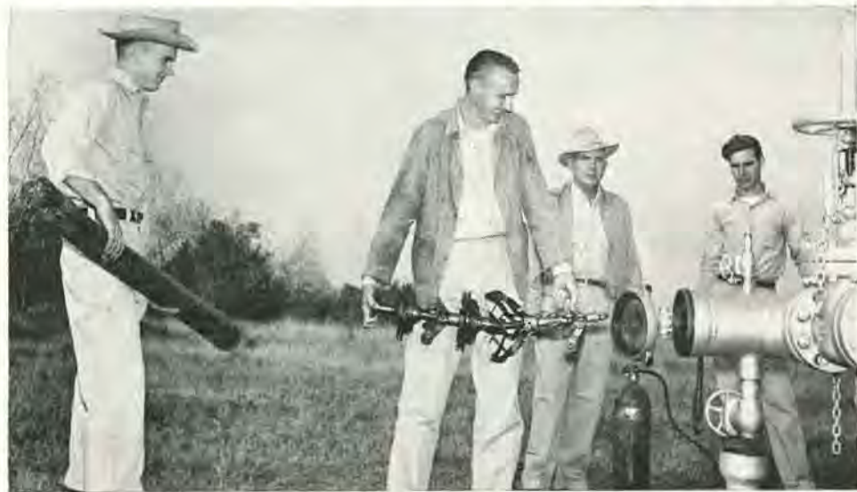
The Baytown Maintenance crew prepares to start a scraper-type go-devil. Holding it is J. H. Stark with J. D. Andersen ready to seat it in the pipe with a log. C. C. Moss, foreman, and J. S. Broomas are ready to assist in safety measures.
