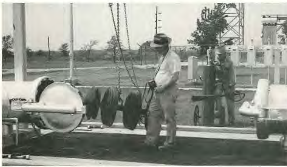
L. L. Arnold, Garfield Station assistant chief engineer, puts a plug-type cleaner into the 24-inch Rancho Pipe Line System while checking a gas detector in his right hand. The man manning the fire extinguisher is R. D. Webb, utilityman.
